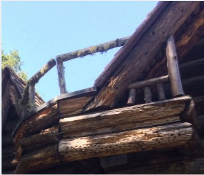
The Log Cabin is in a such a state of severe disrepair, it may not be possible to rehabilitate it in its current form
