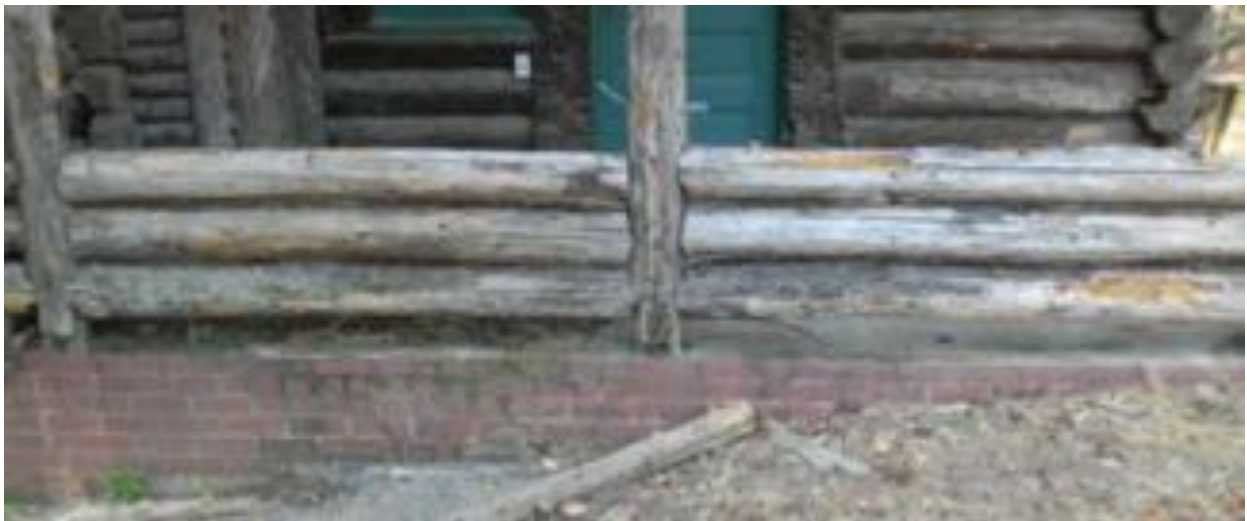
Fig.45 – Log conditions at rear porch
