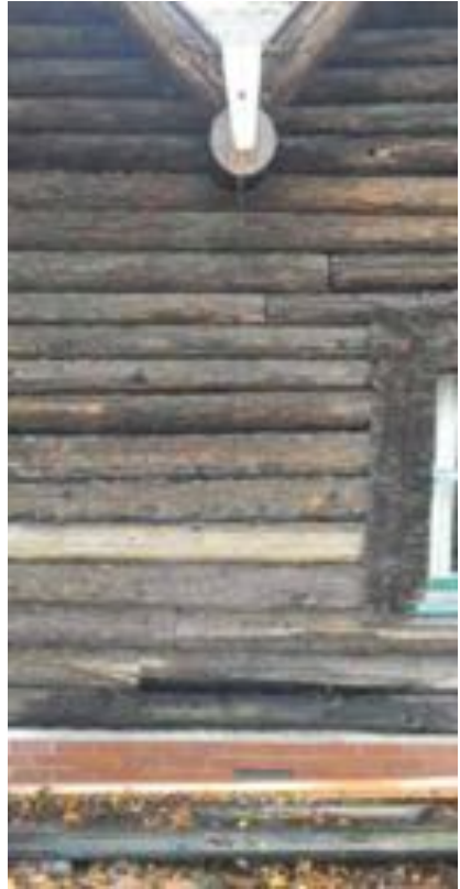
Fig.38 – Log and roof drainage conditions at west side
