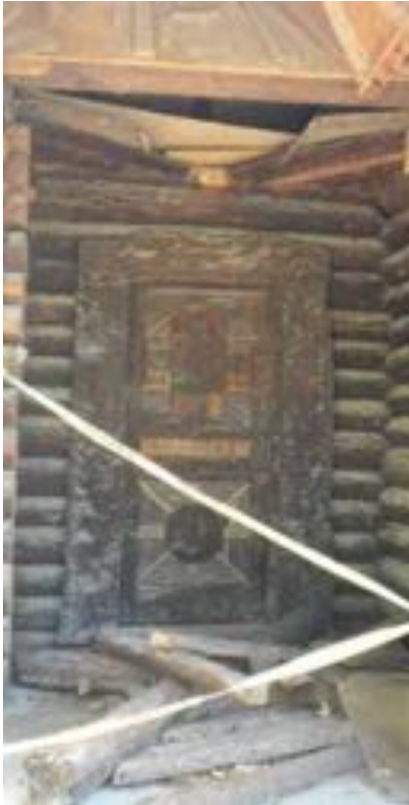
Fig.39 – Structural conditions at front porch and entry door
