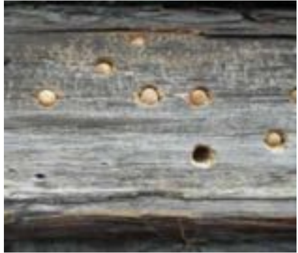
Fig.43 – Log conditions at west side wall
