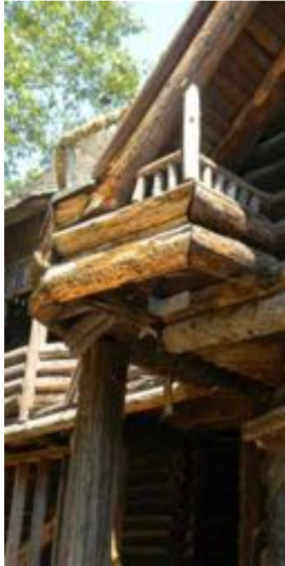
Fig.37 – Log conditions at front gable ornamentation
