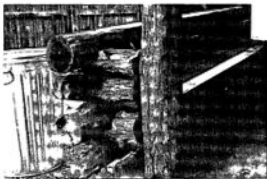
Log bases and ends show severe water, fungus, and termite damage.
