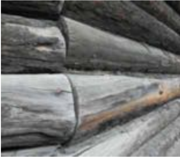
Fig.42 – Log conditions at east side wall
